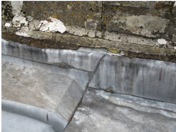
Fig.9 Defective pointing to chancel flashings.
