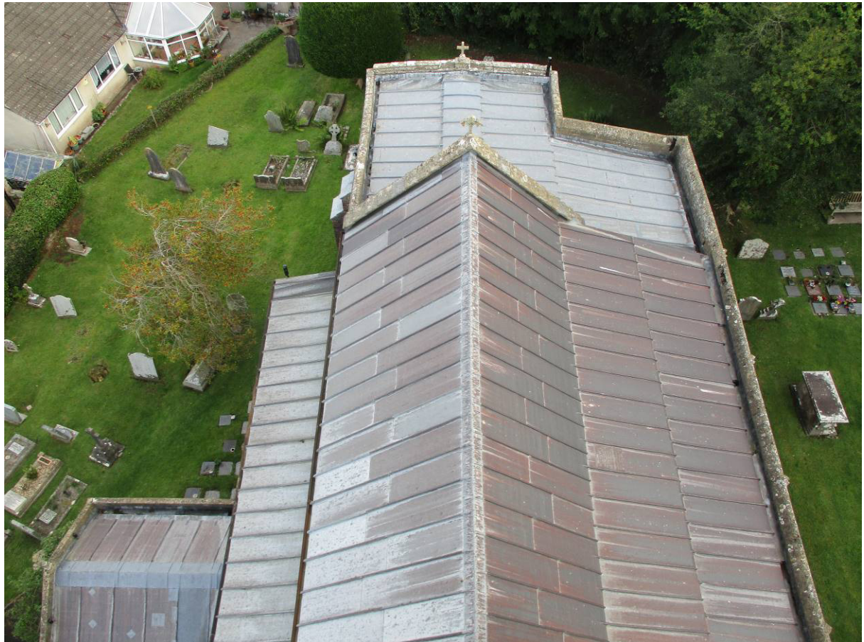
Fig.6 The roof of the nave, chancel, organ chamber, aisles and porch seen from the tower.
